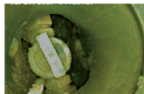
Non-Lead Service Line
